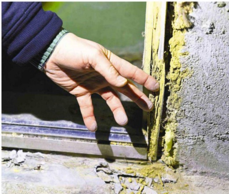
A home inspection revealed past termite dirt and rot at a home in Huntington Station.
