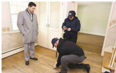
During the inspection, Rob Byrne shows Douglas Elliman's Michael Furino a damaged floor board while Taiysha Vargas takes notes.
