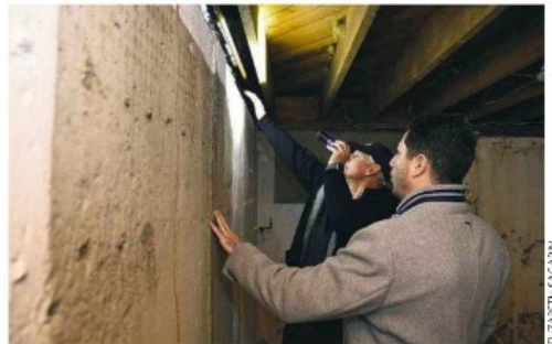
Higher Elevation's Rob Byrne inspects the basement of the Huntington Station home with Douglas Elliman's Michael Furino.
